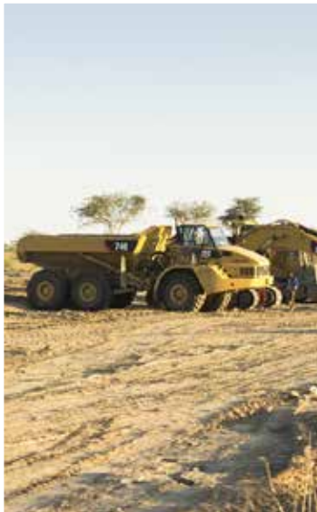
The upgrading of Trunk Road 1/6 between Windhoek and Okahandja commenced in 2014 and is expected to be concluded in 2019, with an estimated total cost of N$3,081 billion.
